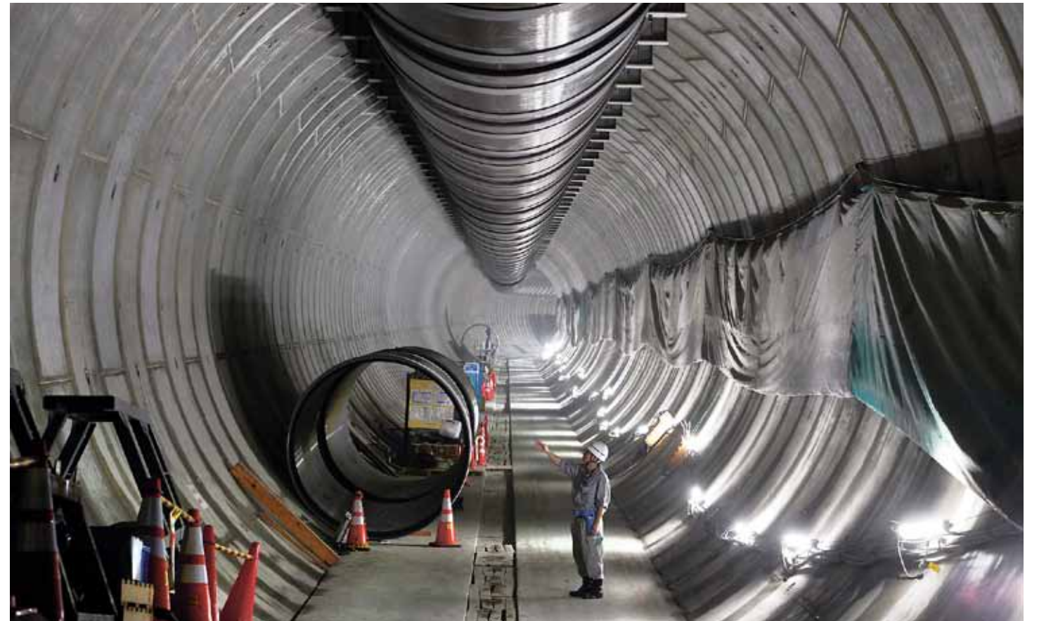
A worker points to the wall of a section of the Furukawa reservoir project being built in central Tokyo on Aug. 7. When completed in 2016, the 3.3-km-long subterranean reservoir will be able to hold 135,000 cu. meters of water, enough to fill 54 Olympic-sized swimming pools. BLOOMBERG
